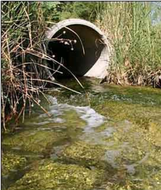
A dewatering pipe in one of the area tributaries. Photo provided by Nick Rice, SNWA
